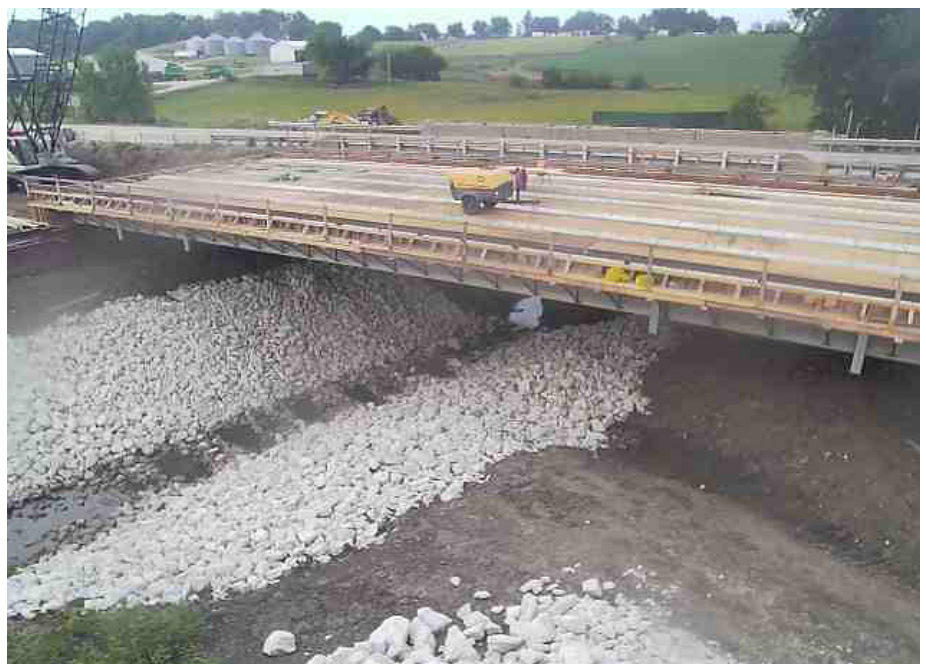
Slide-in bridge during accelerated bridge construction next to the original IA 92 Massena Bridge
