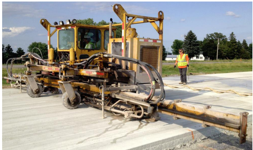
Non-typical conventional gang-saw machine used at one site
