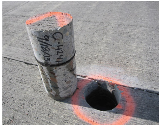
Sample core retrieved in 2013 showing the relationship to Joint 4241 Cell 505 with its fabric bond-breaker
