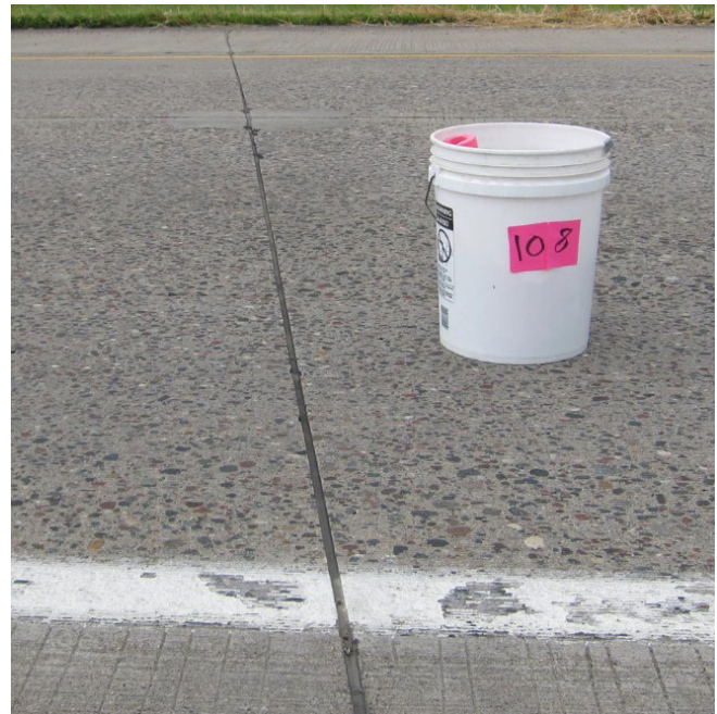
Sample core retrieved in 2013 showing the relationship to Joint 4241 Cell 505 with its fabric bond-breaker
