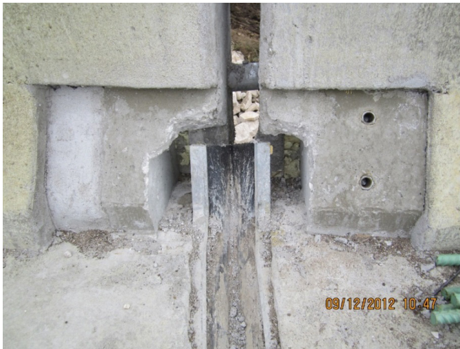
Field construction of strip seal termination turn-up at barrier rail with blackout
