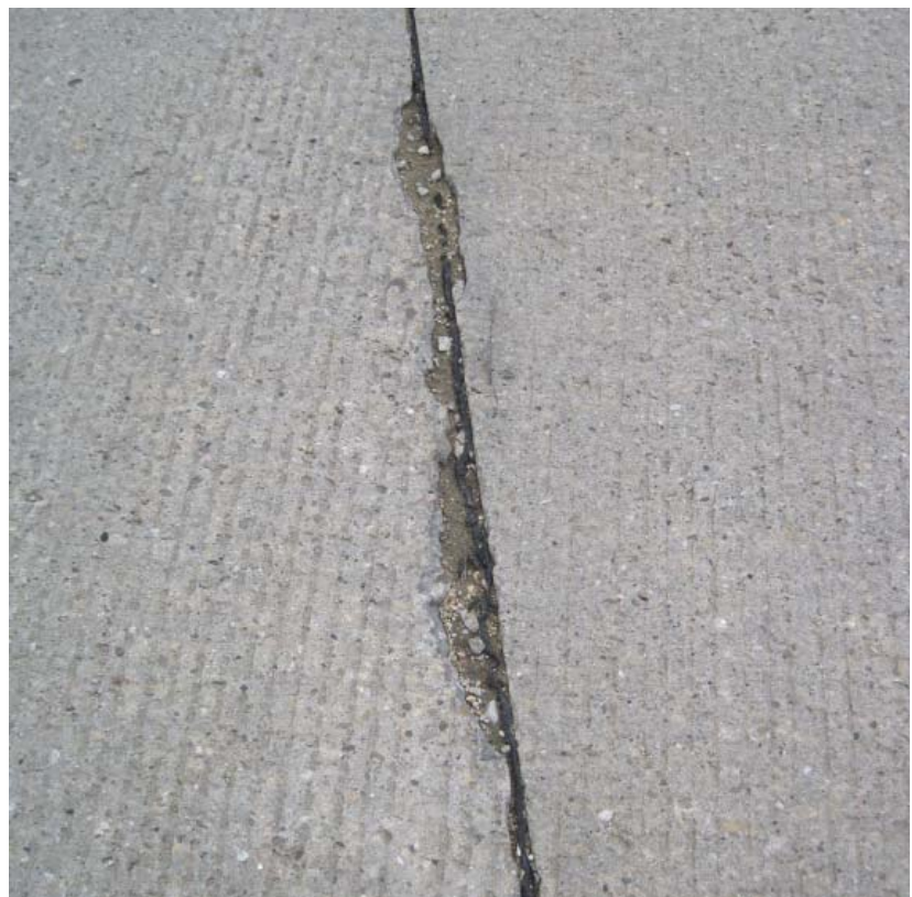
Figure 1. Premature joint distress (photo courtesy of Jim Grove, FHWA)
