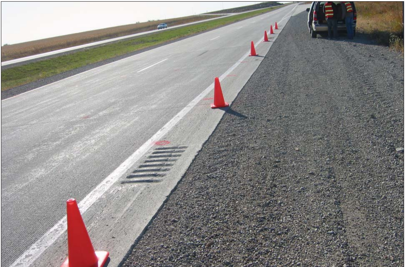
Pavement surface distortion caused by settlement, Highway 18 east, Iowa
