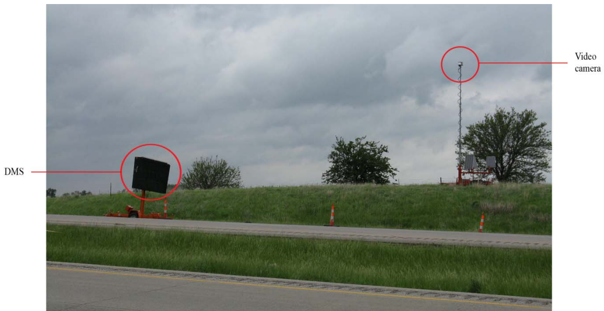
Figure 4. Typical installation (may include the DMS, left, and sometimes a solar-powered video camera, right) (photo courtesy of Iowa DOT)
