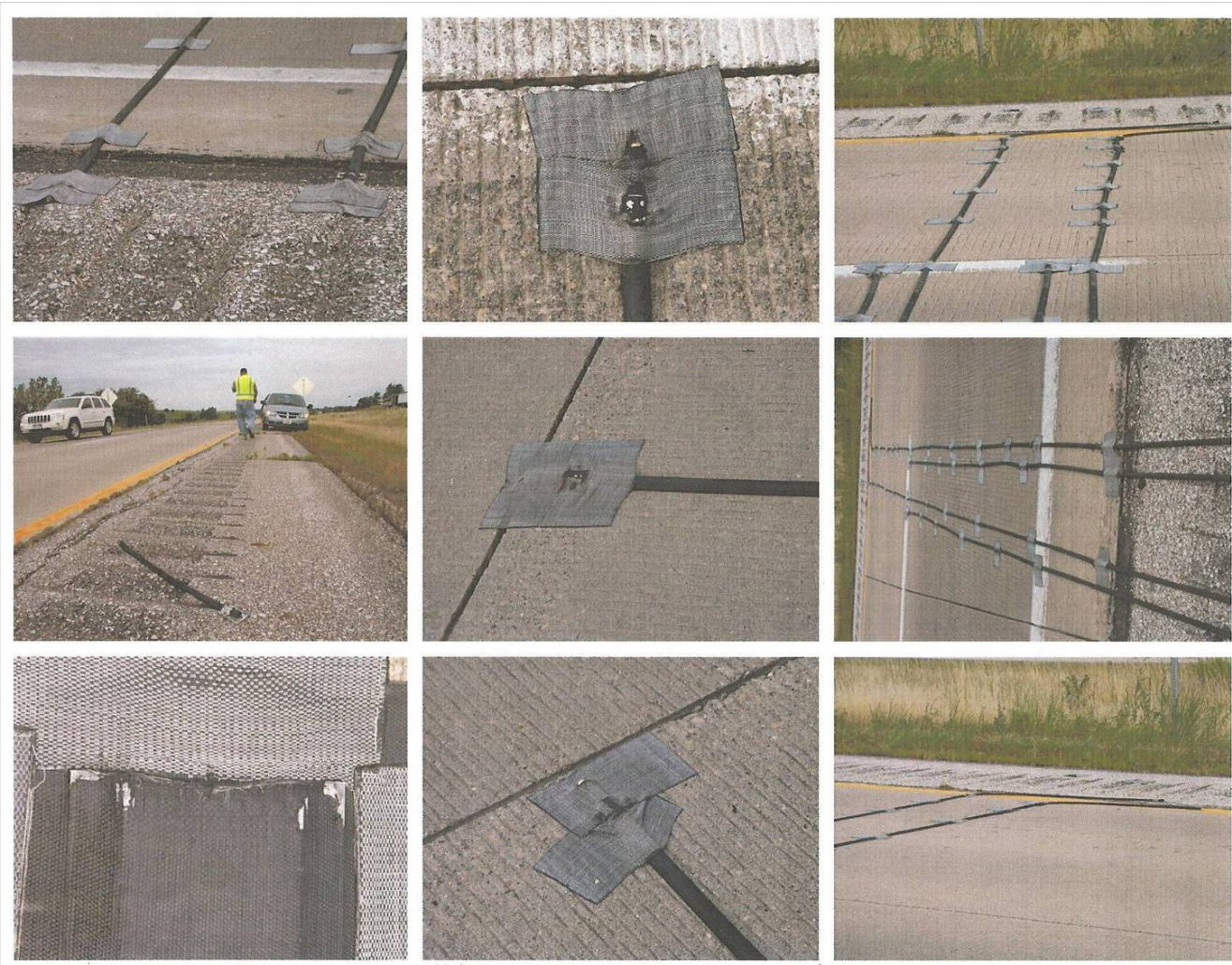
Figure C.1. Photos of damaged tubes, tape, and hold-down devices (photos by Brad Greffe)
