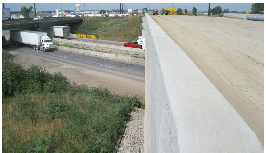
One of five bridges that had strain gauges installed on the decks and girders at several transverse sections for field tests and inspections
