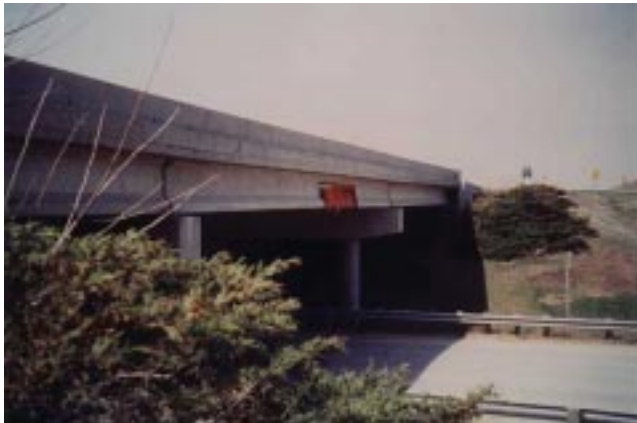
FIGURE 1 Elevation view of WB bridge, looking West (damaged Beam 1W in center span)
