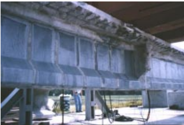
FIGURE 9 Beam 2W after repair with CFRP longitudinal plates (not shown) and CFRP stirrups
