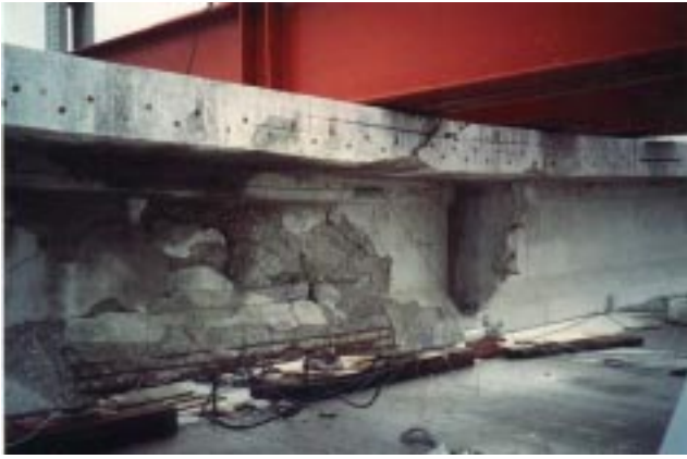
FIGURE 8 South face of Beam 1W in the damaged region following the ultimate load test
