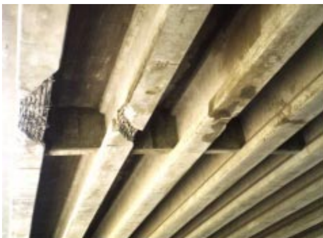
FIGURE 2 Underside of damaged WB bridge, Beam 1W on left
