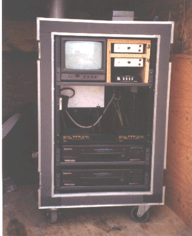
Figure 4-2 View of Electronic Equipment in a Data Collection Trailer
