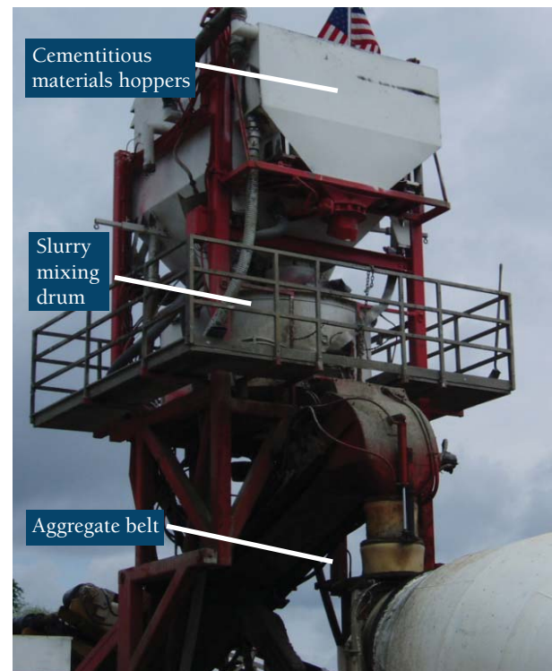
Components of the two-stage mixing tower at the Minnesota research site
