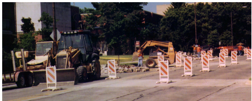
Typical traffic control devices near work zone
