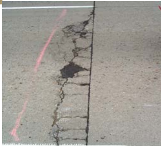
Dowel Bar Misalignment
