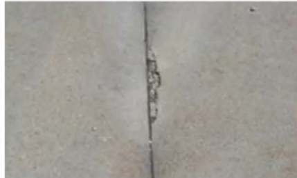
Figure 11 – Image of incompressible damage to concrete joint (Photo credit CP Tech Center)
