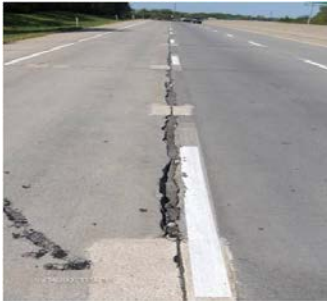
Freeze Thaw Damage
