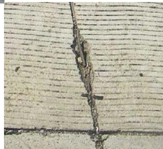
Incompressible Joint Damage
