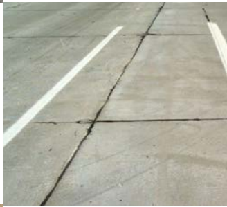
Early Saw Joint Raveling
