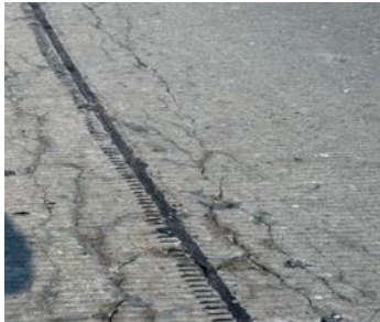
Saturated Joint with Unsound Aggregate
