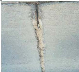
Saturated Joint Backer Rod Damage
