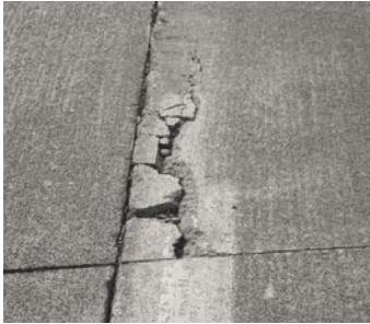
Deflection Spalling From Heavy Vertical Loads
