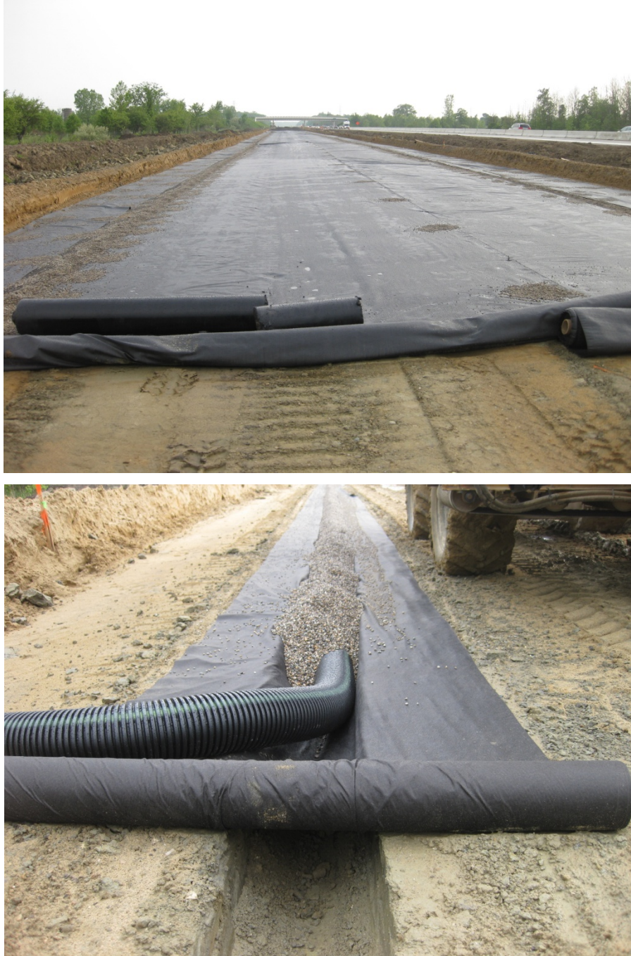
Figure 7. Geoturf ® W270 woven geotextile separator installed on top of the subgrade (top) and longitudinal trench drain wrapped around a non-woven geotextile and porous backfill material (bottom)
