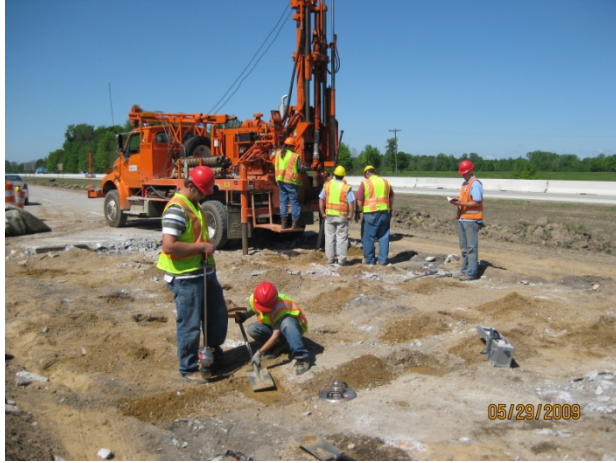
Figure 75. TS2-B: Preparing test locations for in situ testing (foreground) and the MDOT drilling rig obtaining Shelby tube samples
