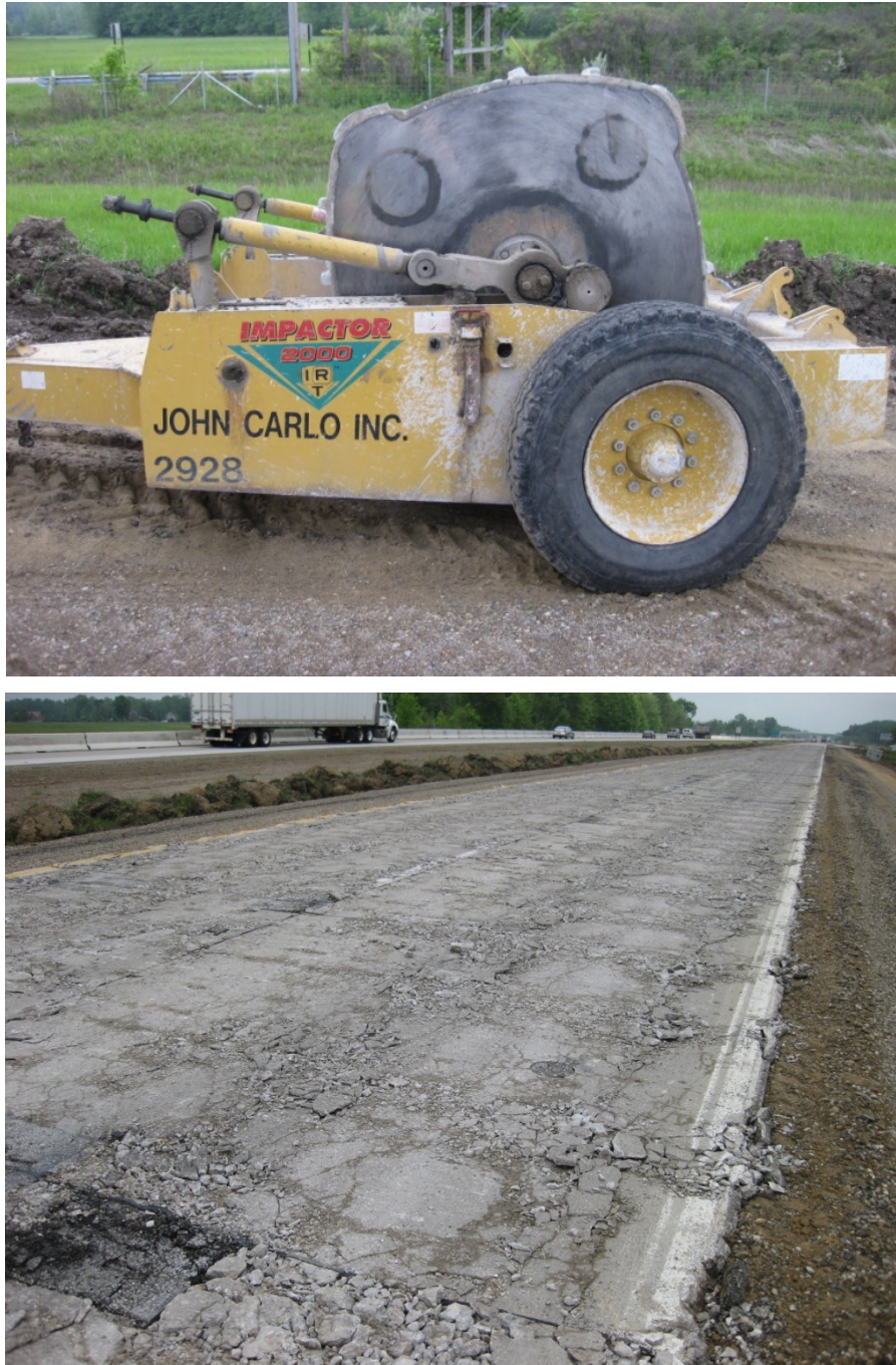
Figure 5. Four-sided impact roller used to break the existing pavement layer (top) and pavement surface after impact roller passes (bottom)
