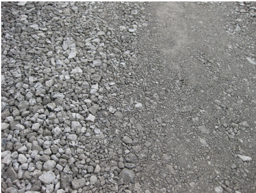
Figure 9. OGDC base layer before trimming (top) and a close-up view of the OGDC base layer after trimming and compaction (bottom)
