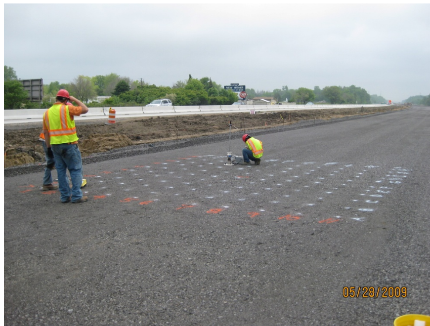
Figure 52. TS1-B: Photograph showing testing on the 0.6 m x 0.6 m grid pattern
