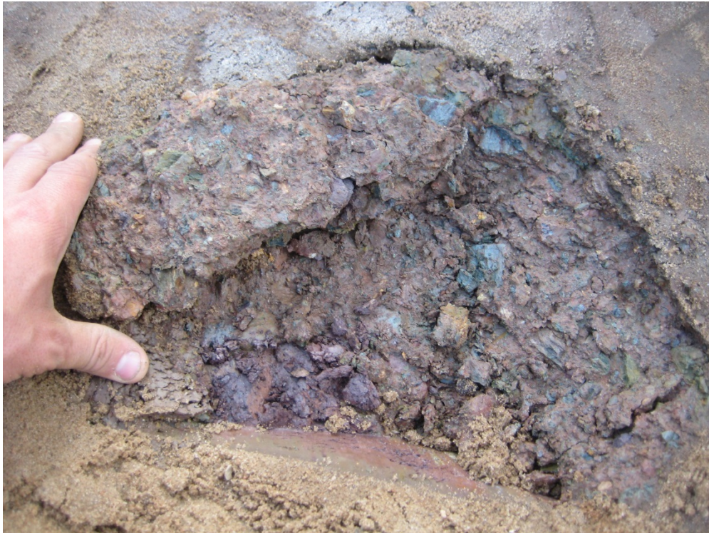
Figure 35. TS1-2: Excavation through the thin sand subgrade layer for tests on the subbase
