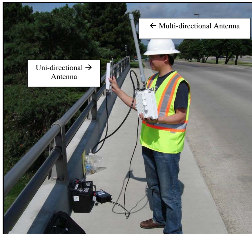
FIGURE 2 Mesh Router with Multi-directional and Uni-directional Antenna
