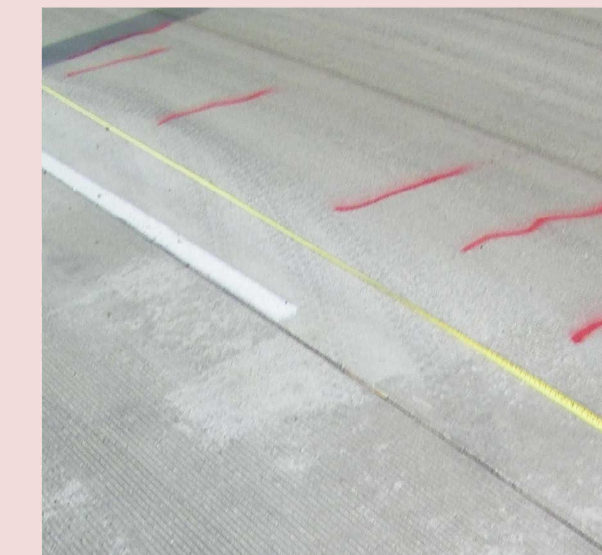
Frequent wide cracks under wheel path, and surface wearing
