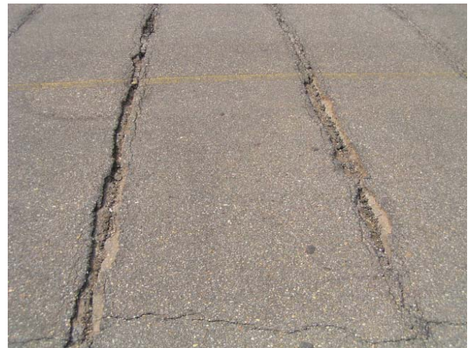
Figure 8. Butler County Bridge wearing surface cracking.
