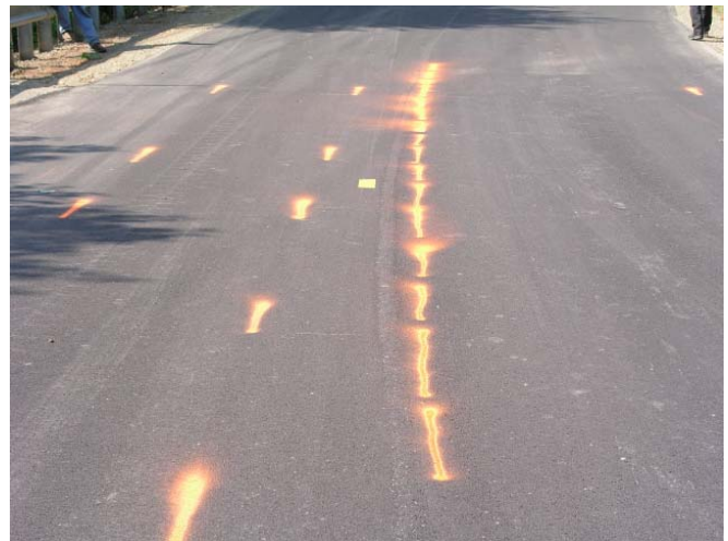
Figure 14. Angelica Creek Bridge 2003 wearing surface.
