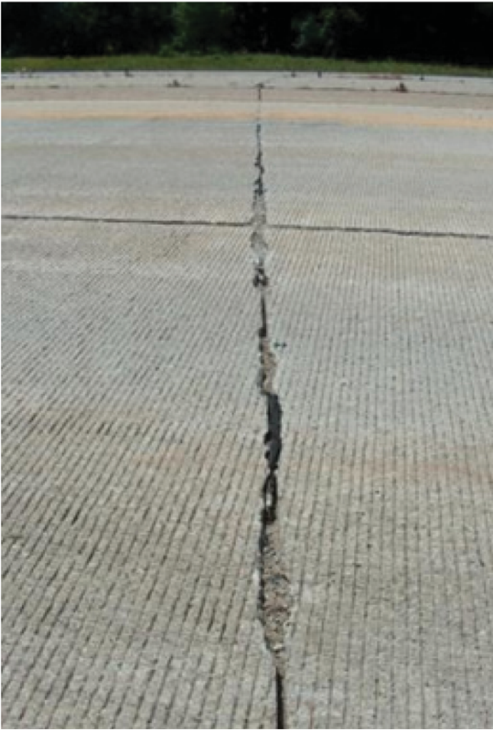
Figure 4. Typical mechanical distress
