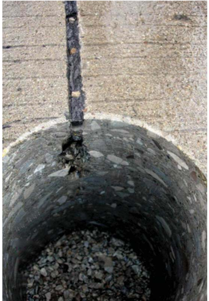
Figure 5. Example of damage occurring in a slab that has not cracked out
