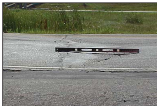
Figure 1. Deteriorated pavement that is a good candidate for FDR
