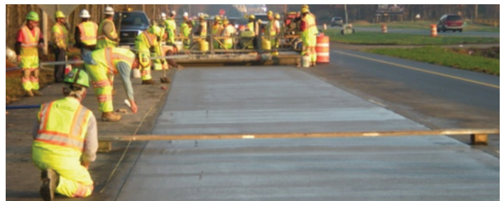
Construction of small concrete overlay project using transit-mixed concrete and hand placement methods on US-13, Delaware
