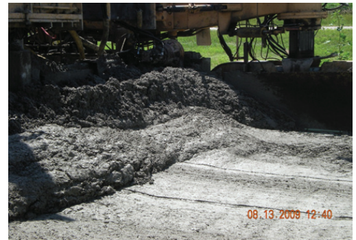
Concrete head in front of paver during construction of unbonded concrete overlay over concrete pavement, Route 50, South Dakota
