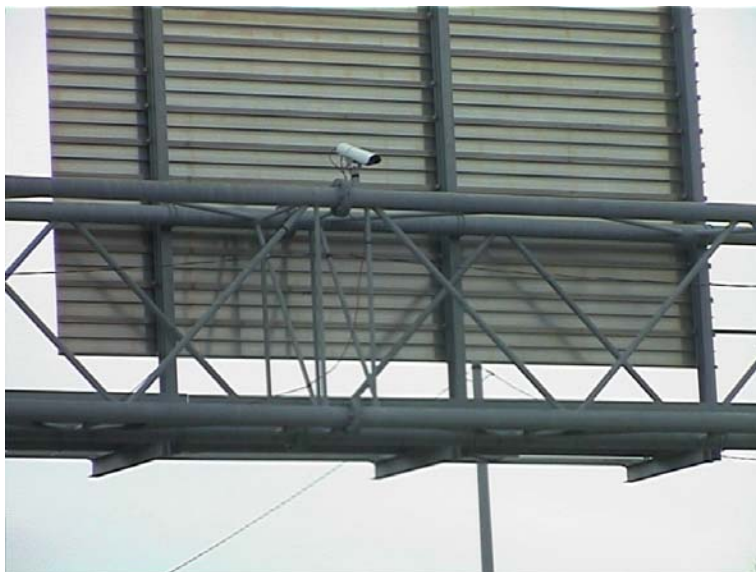
Figure 3. WZSAS Camera Mounted Above Roadway.
