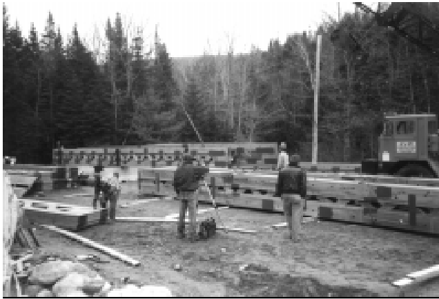
Construction of the Byron bridge. Galvanized MPC (G90) joints are painted with an epoxy paint to add corrosion resistance.
