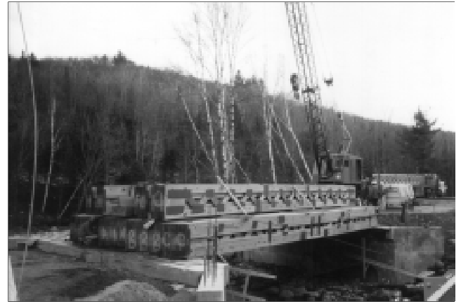
Construction of the Byron bridge. Packets of 10 to 20 trusses lifted in single units.
