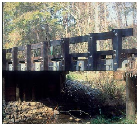
This timber bridge located in Putnam County has a stress-laminated deck, 30-feet long by 16-feet wide, constructed from southern yellow pine and treated with Pentachlorophenol.
