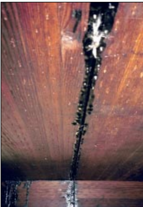
Figure 5. Paving membrane leakage.
