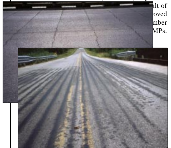
Figure 4. Bleeding caused by over treatment (note tracking from bridge to approach).
