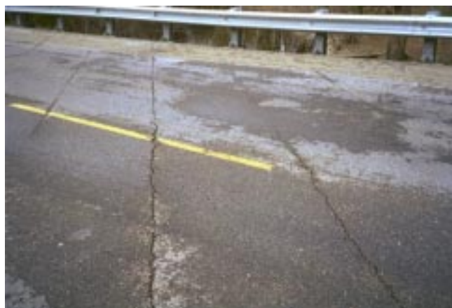
Figure 1. Pavement cracking caused by differential deflection of panels.
