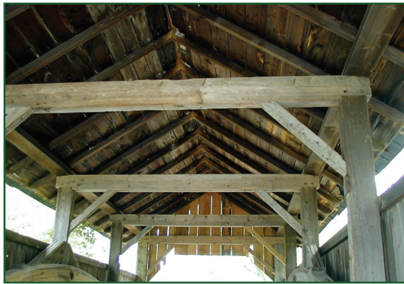
In covered bridges, naturally durable wood species are an attractive option for replacement components that are protected from moisture
