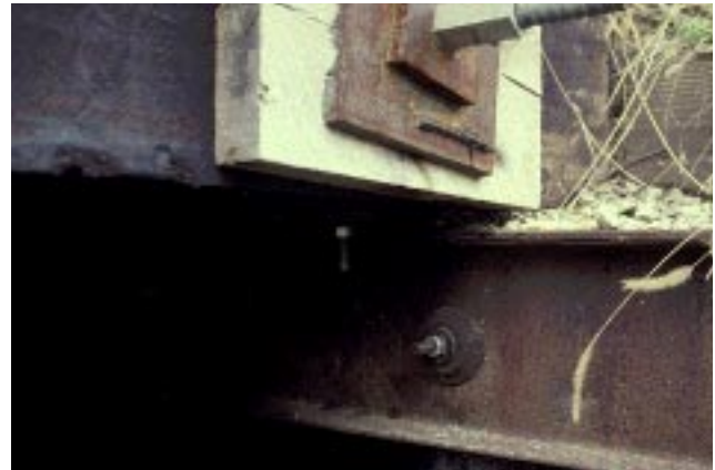
Figure 20—(top) Schematic of west abutment of Decatur bridge. The edges of the deck curve upward away from abutment; (bottom) gap between abutment and deck at the northwest corner of the Decatur bridge.
