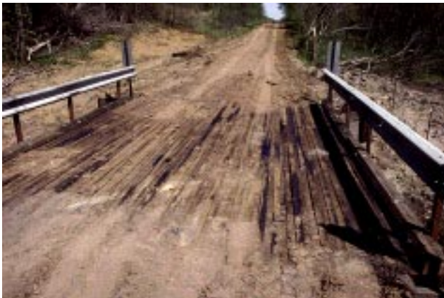
Figure 22—Uneven deck surface of the Hibbsville bridge as a result of unequal depth of the laminations.
