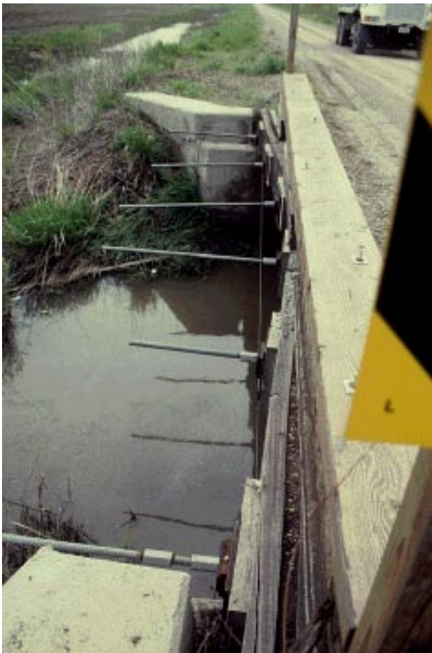
Figure 19—Distortion of north edge of Dean bridge. The width is approximately 216 mm (8.5 in.) narrower at the midspan than at the abutments.
