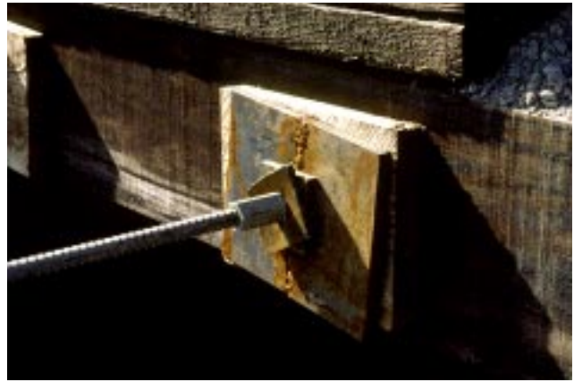
Figure 24—Two steel plates butt jointed and welded together to form bearing plate at the Dean bridge.
