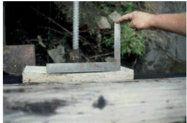
Figure 23—Top view of white oak bearing plate deformation in the Decatur bridge.
