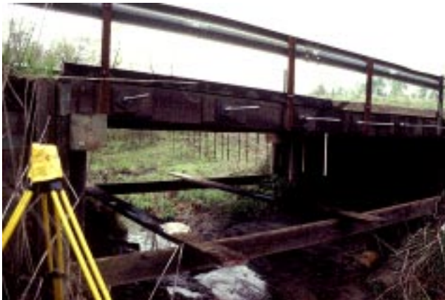
Figure 8—Load test deflection measurements were obtained by reading values from calibrated rules suspended from the underside of the deck with a surveyor's level. Load test 2 of the Hibbsville bridge is shown.
