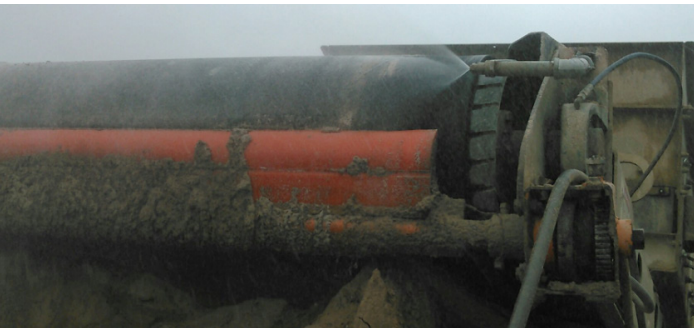
Figure 3. Water spray dust suppression system on concrete crusher (photo courtesy of Duit Construction)
