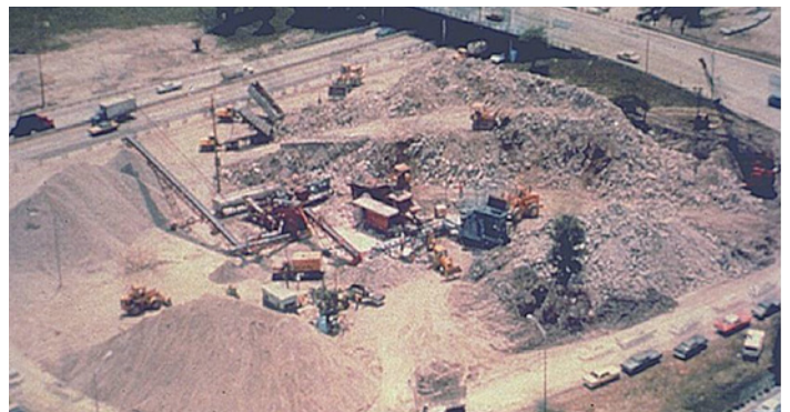
Figure 4. Concrete recycling operation set up inside of Edens Expressway cloverleaf interchange (photo from NHI 1998,
