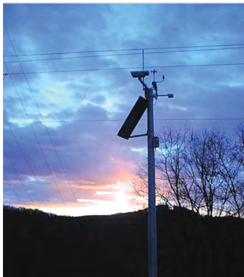
An RWIS site in Minnesota.
