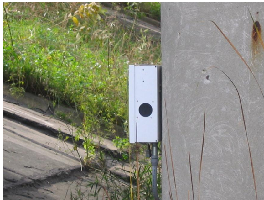
Figure 5. Lockable box with 12 V power supply located under the bridge
