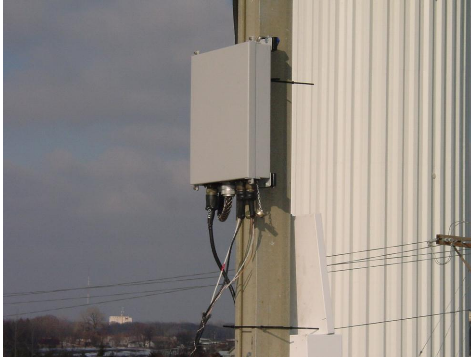
Figure 3. Electronics module mounted to the side of the pole
