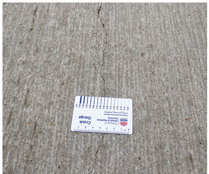
Figure 64. Concrete pavement with fibers and hairline crack
