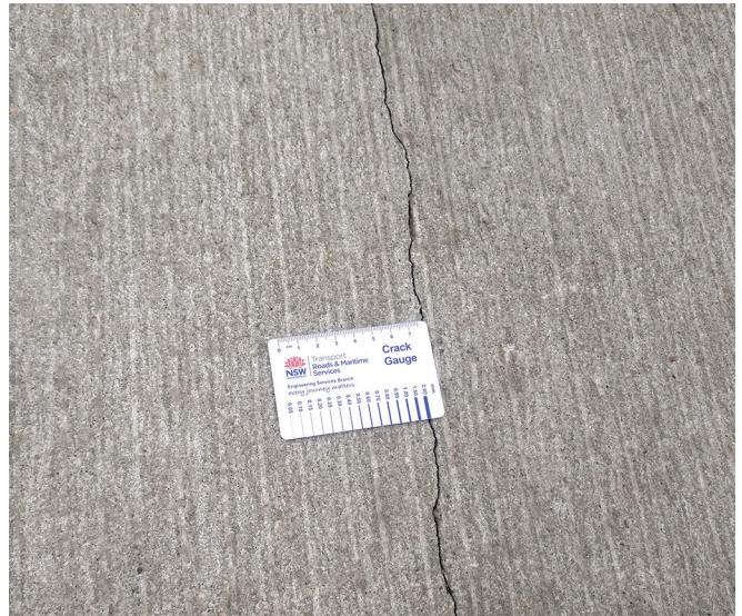
Figure 63. Concrete pavement without fibers and with noticeable longitudinal crack
