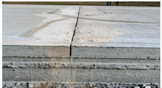
Figure 35. Activated transverse joint
