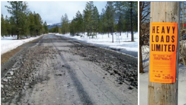
To prevent excessive roadway damage during spring thaws, DOTs apply spring load restrictions
