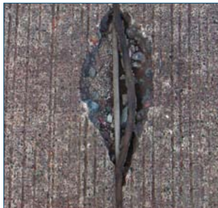
Localized damage on each side of a joint
