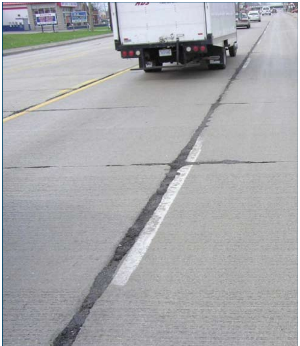
Distress in a longitudinal joint on a city street
