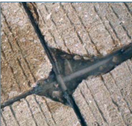
Water ponding at joints
