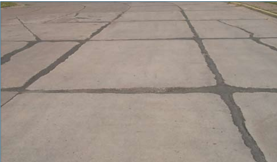
Distress in longitudinal and transverse joints
