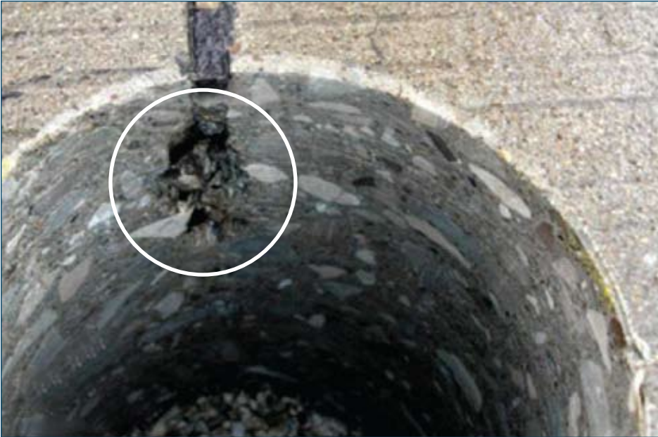
An example of damage occurring below the backer rod
