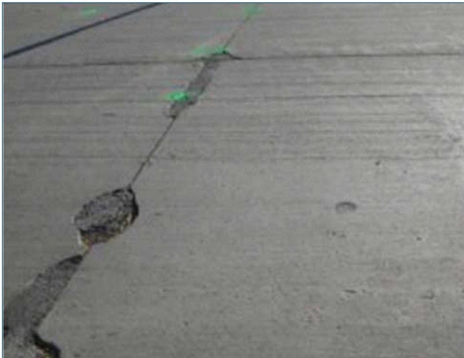
Loss of material
