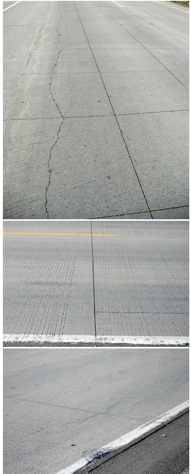
Armen Amirkhaniyan, used with permission (top); Matt Zeller, Concrete Paving Association of Minnesota, used with permission (center and bottom)
