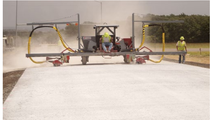
Brent Burwell, ACPA, OK/AR Chapter, used with permission Figure 19. Span saw used to cut transverse contraction joints at 6 ft center on center
