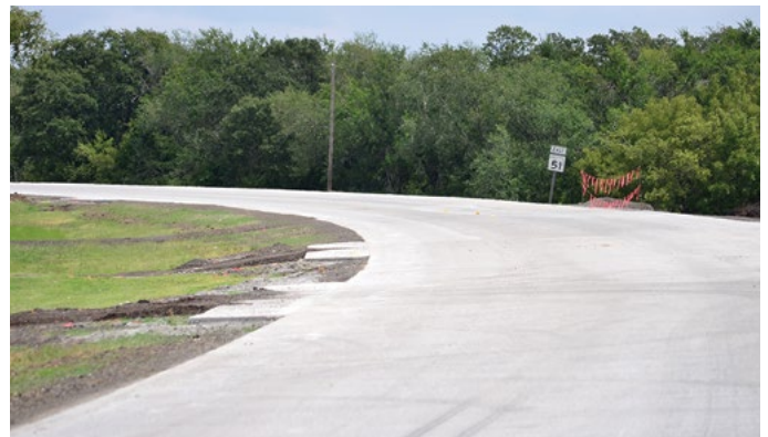
ACPA, used with permission (Duit Construction Company, Inc.) Figure 20. Completed concrete overlay, with drainage structures extended to accommodate widening of the existing roadway
