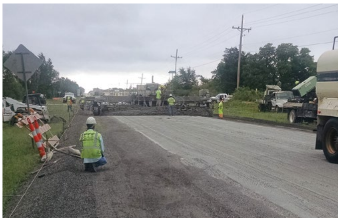
ACPA, used with permission (Duit Construction Company, Inc.) Figure 18. Roadway closed to through traffic during construction, allowing full-width paving of the concrete overlay and significantly reducing the construction duration
