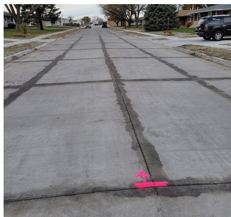
Phase 3 sealer application on SE 8th Street in Ankeny, Iowa, for longer term field evaluation
