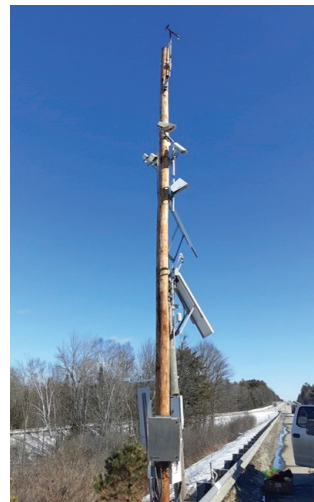
Stationary friction sensors mounted at an RWIS site in Etna, Maine
