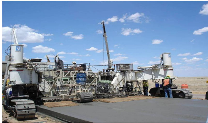
1 st CDOT Paving Project w/ PLC US 287 (Ports to Plains route) in eastern CO
