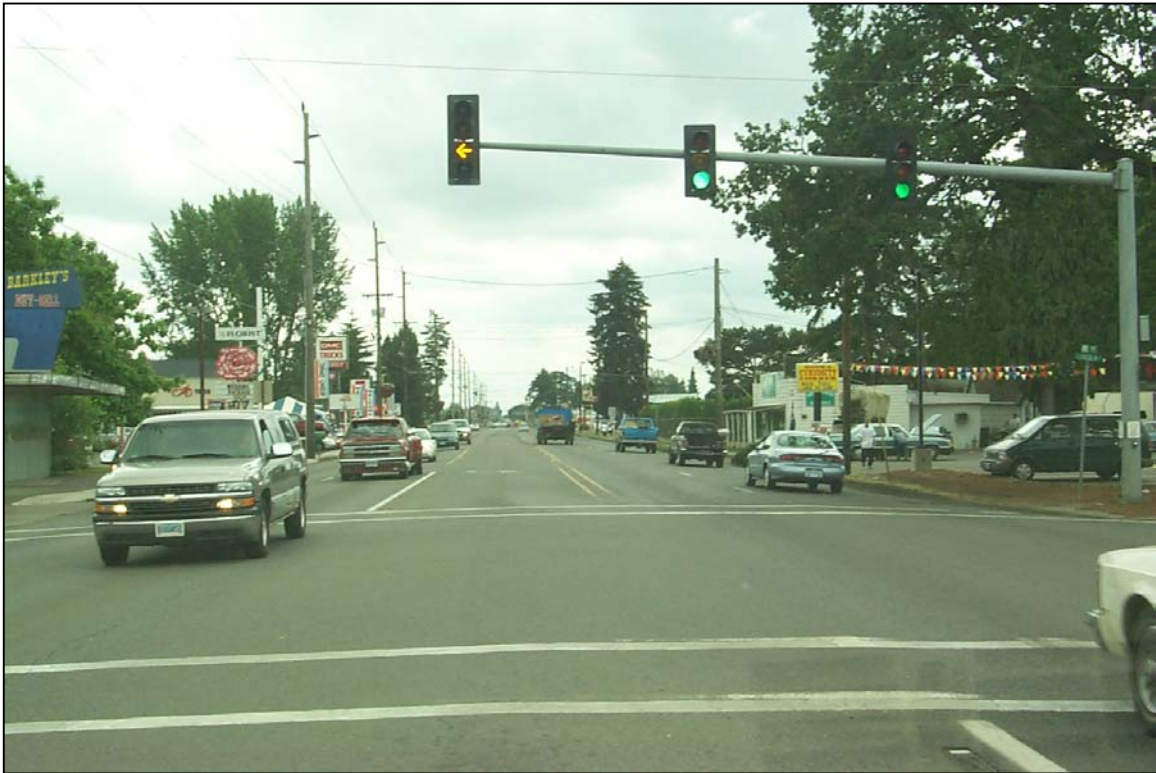
FIGURE 5. Four-Section Vertical Flashing Yellow Arrow Permissive Indication
