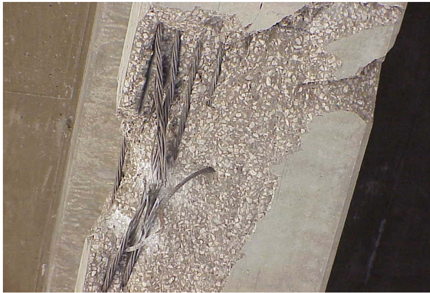
FIGURE 3. Photograph of the Damage to Beam 2 in the Altoona Bridge
