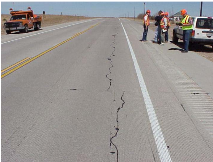
FIGURE 7. Wandering Cracks in the Northbound Lane of US-287
