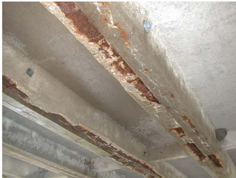
FIGURE 4. Typical PCB Deterioration
