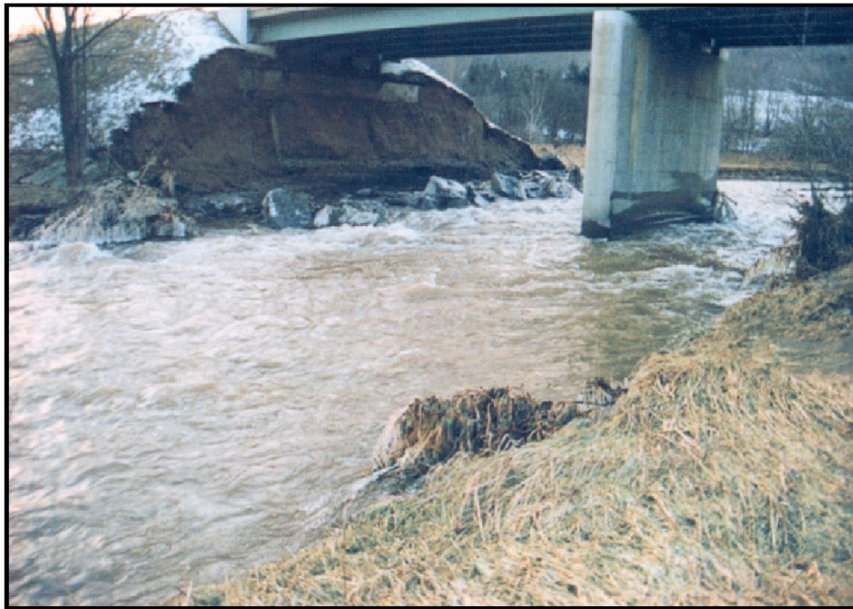
Figure 1. Scour-induced failure of the earth-fill embankment at a spill-through abutment
