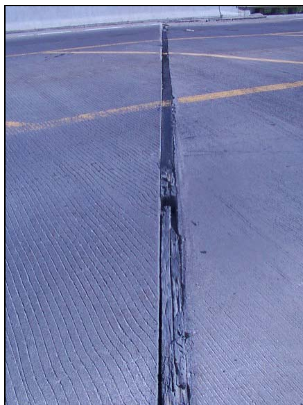
(a) Deteriorated joint filler (Bridge No. 2034.20035, District 5)
