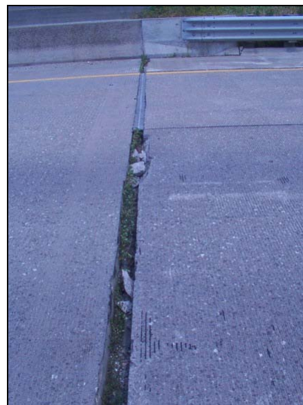
(b) Missing joint filler (Bridge No. 9265.7L218, District 5)
