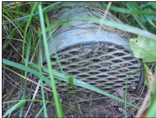
Figure 2. Example of a blocked subdrain outlet (Bridge No. 9266.2R218, District 5)
