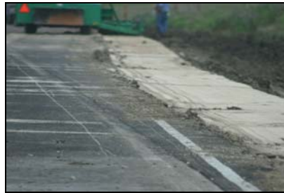
Figure 5. Edge line damage due to shoulder maintenance
