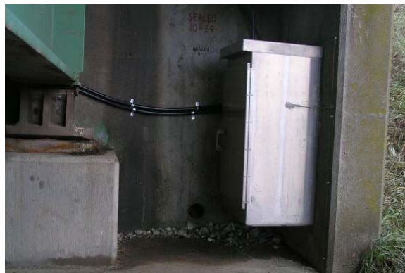
Figure 7. Aluminum cabinet mounted on the north corner of the west abutment wing wall
