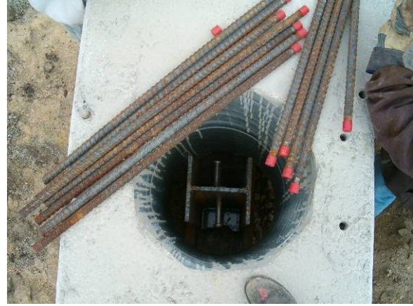
Figure 6. Abutment CMP blackout
