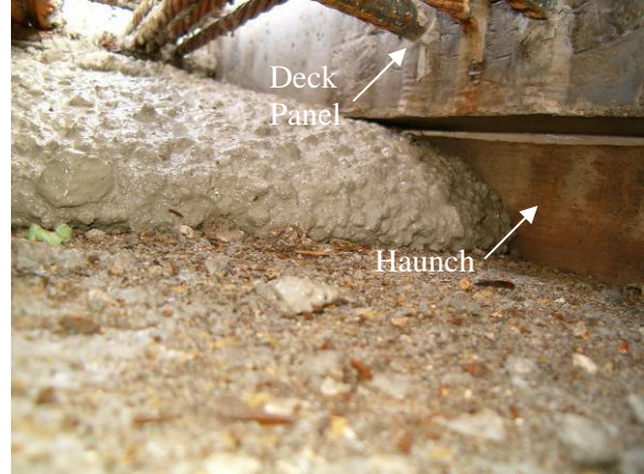
Figure 12. Concrete consolidation in haunch
