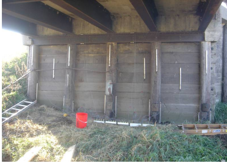
Figure 2. Timber substructure instrumented with strain gauges (south abutment, Bridge No. 237350, Mahaska County)
