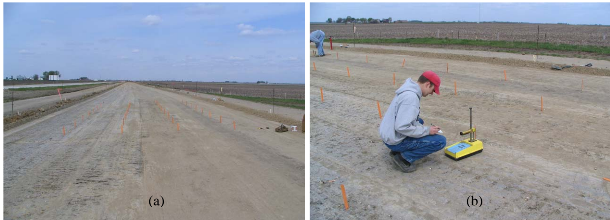
Figure 9. US-20 test site: (a) test grid, (b) nuclear moisture density gage testing
