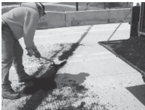
Rubber particles are spread and then sealed into the expansion joint. Photo courtesy of the Iowa DOT.
