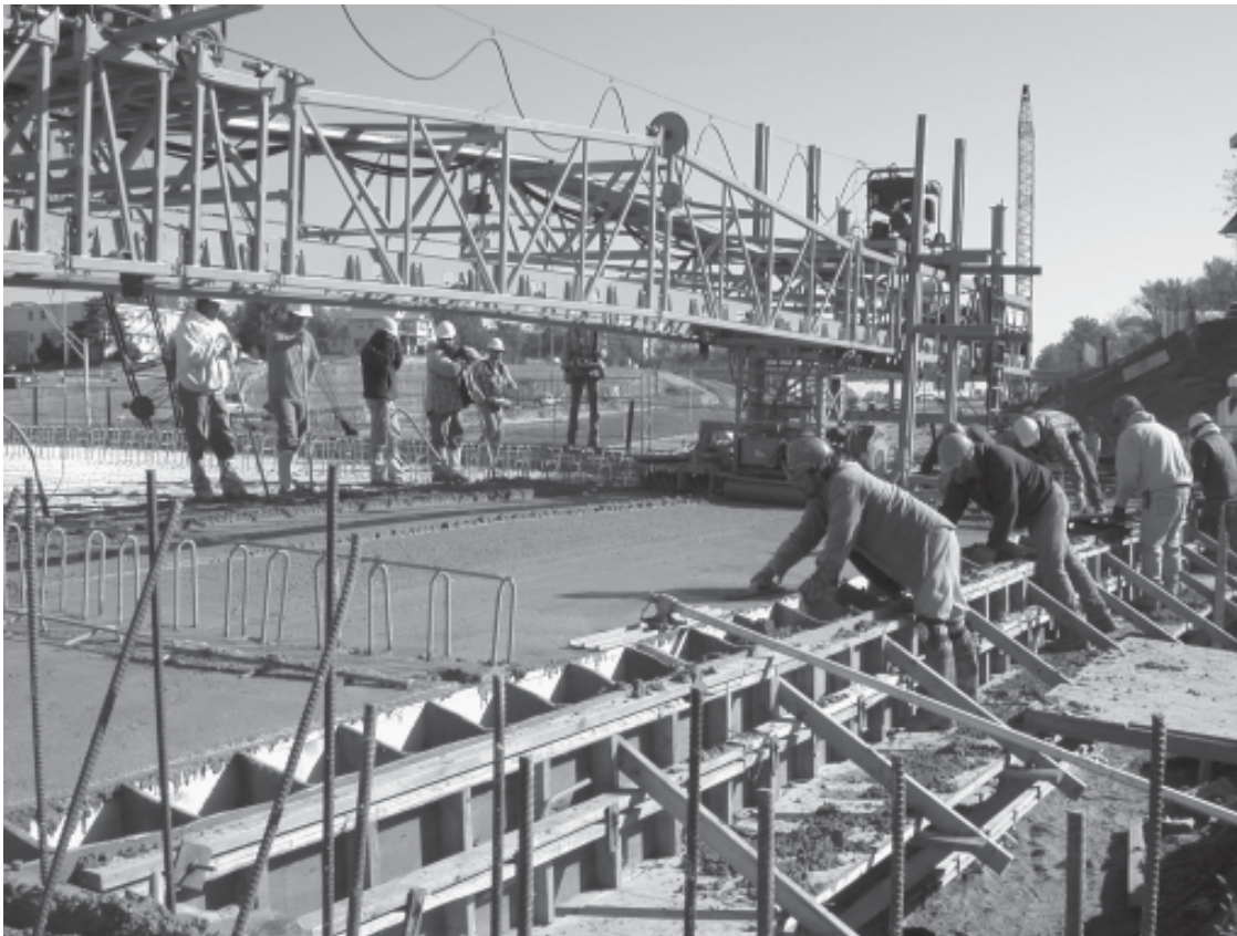
East 9 th Street, Des Moines, bridge deck pour: finishing machine and crew, October 2002. Photo courtesy of Kenneth Dunker, Iowa DOT.
