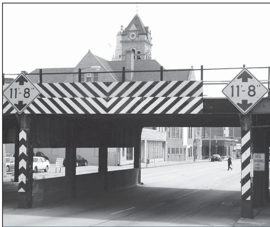
CARS reduced crashes of over-height vehicles by 50 percent at this low-clearance railroad bridge in Scott County. They installed warning signs, an early detection system, and re-routed vehicles that wouldn't fit under the bridge.
