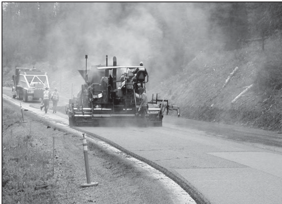
Conventional hot-mix asphalt placed at 320° F, Yellowstone National Park. (Photo courtesy of Dave Newcomb, National Asphalt Paving Association)
