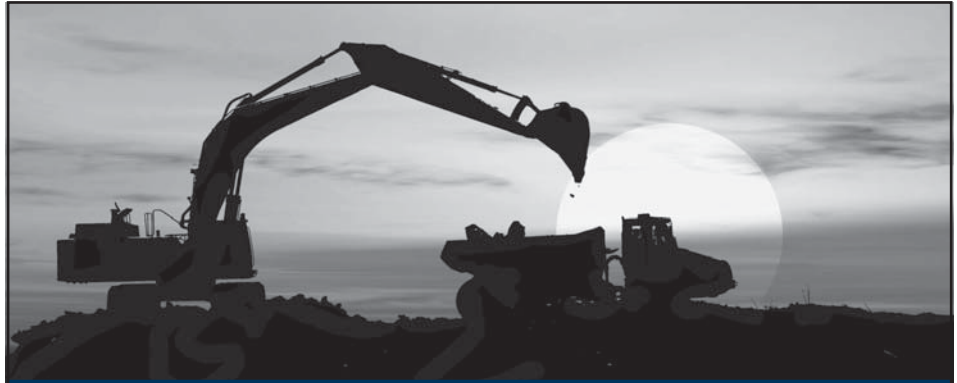
Excavation and trenching are among the most dangerous construction operations.
