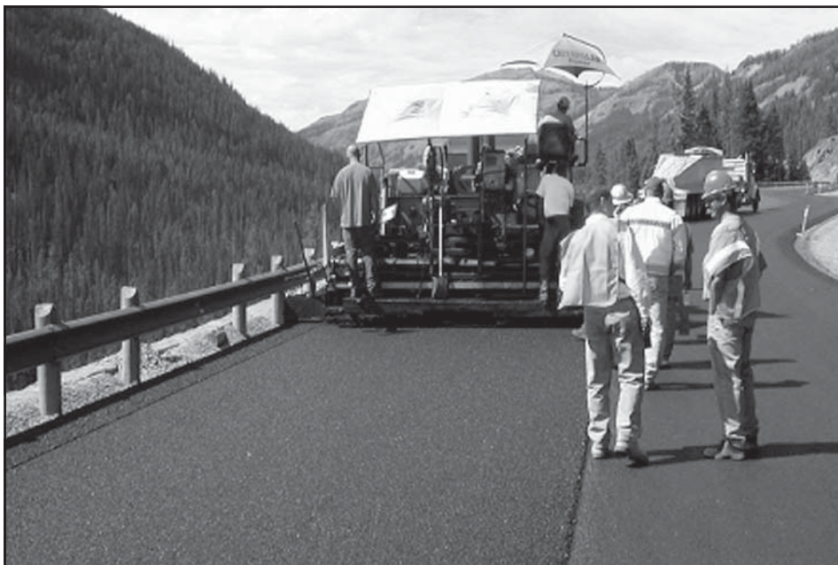
Warm-mix asphalt placed at 245° F, Yellowstone National Park. (Photo courtesy of Dave Newcomb, National Asphalt Paving Association)
