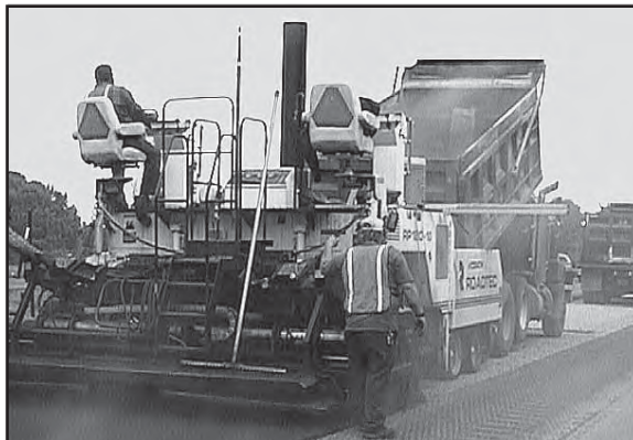
A hot mix asphalt laydown machine with constant flow of materials helps ensure paving uniformity. Photo courtesy of the National Center for Asphalt Technology.
