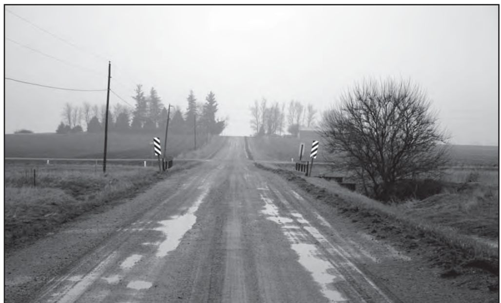
A typical spring gravel road saturated with water and showing signs of distress.
