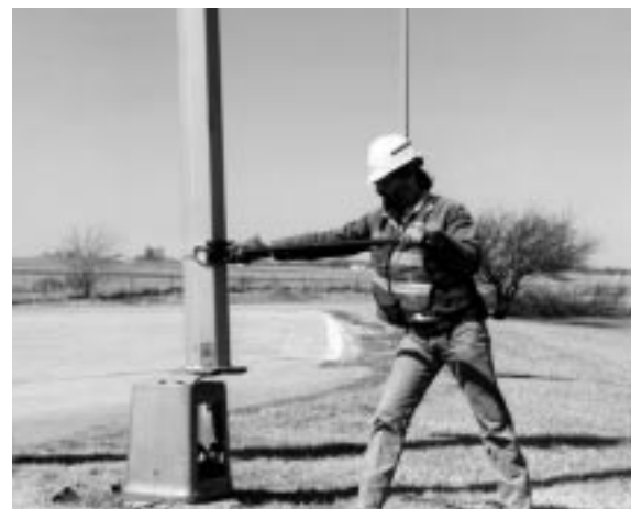
An Iowa DOT employee guides a light pole into place with the pole stabilizer.
