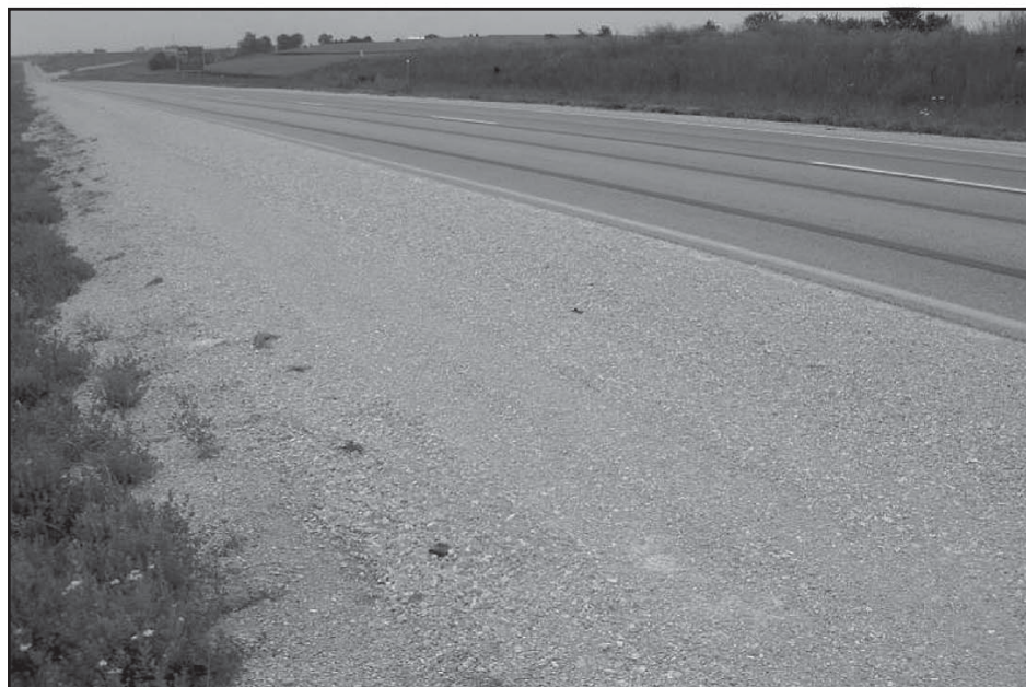
Figure 2. Rutted, unstabilized shoulder (top) Another shoulder area seven months after being stabilized with fly ash (bottom)
