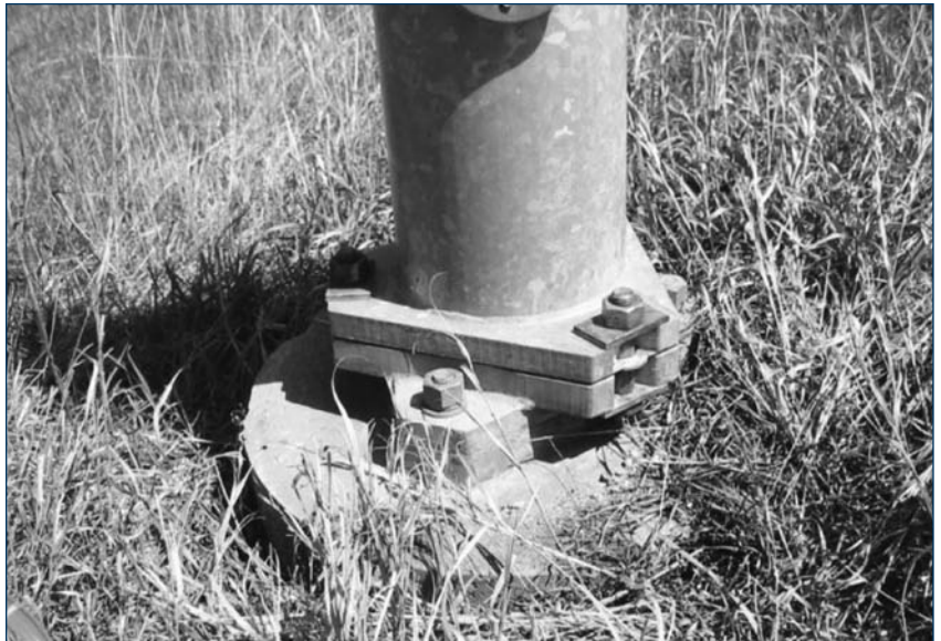
Close-up of a breakaway base on a lighting pole. (Courtesy of the Iowa DOT)
