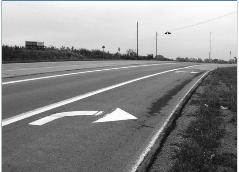
Offset right-turn lane looking northeast along IA-137. (Courtesy of Ryan Pettit, ISU)
