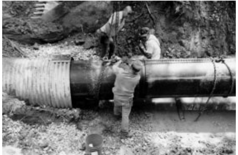
A Hamilton County employee uses a come-along to help snap two sections of liner together.
