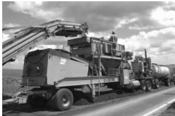
Koss Construction's sizing and rejuvenating portion of the old in-place asphalt recycling train. Photos courtesy of Bryan R. Cawley, ISU research assistant.
